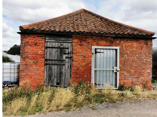
T8b – showing cracks in single storey cowshed from south offering low to medium bat roosting potential (BRP 3-2)
